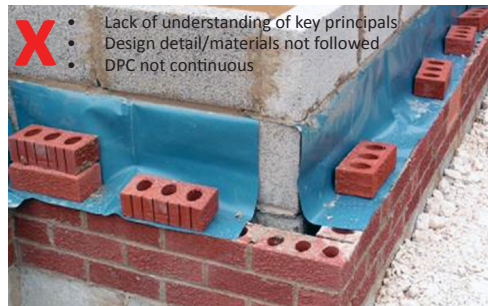
WORKMANSHIP ISSUES WITH FLEXIBLE DPCs
