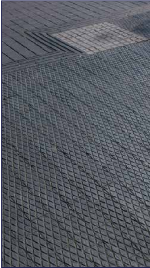
Blue diamond chequer pavers laid in \frac{1}{3} running bond with blue ribbed pavers and blue 2 panel pavers at Camden Lock, London.
