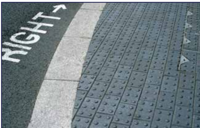
Blue Tactile Blister Pavers in Hammersmith, London.
